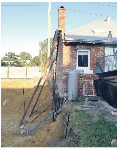
Builder Brad Ross says the property has been shored and propped to prevent further cracking.
